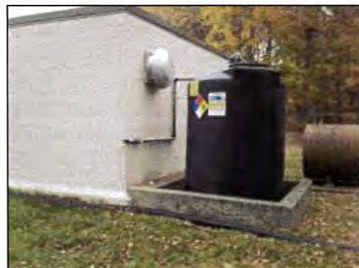
Bioxide Chemical Tank
