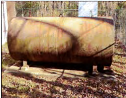
Generator Fuel Tank
