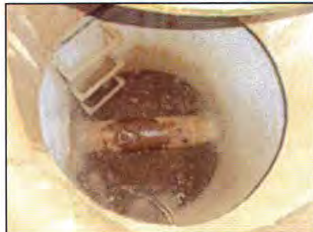
Flow Meter Manhole
