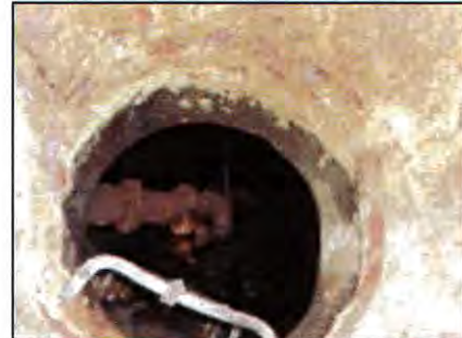
Suction Pipe in Wet Well
