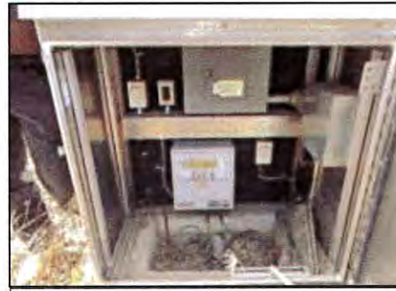
Flow Meter Control
