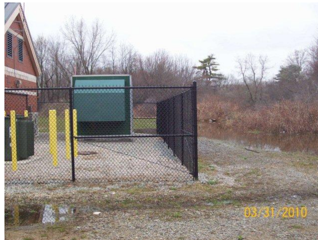
Sandy Bottom Road Pump Station during March 2010 Flooding
